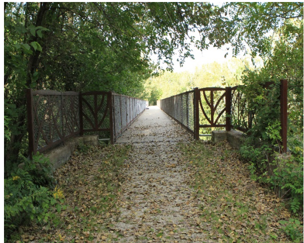
This bridge on the Cedar View Trail is 376' long and spans Cedar Creek. It uses the abutments from an old railroad bridge.
