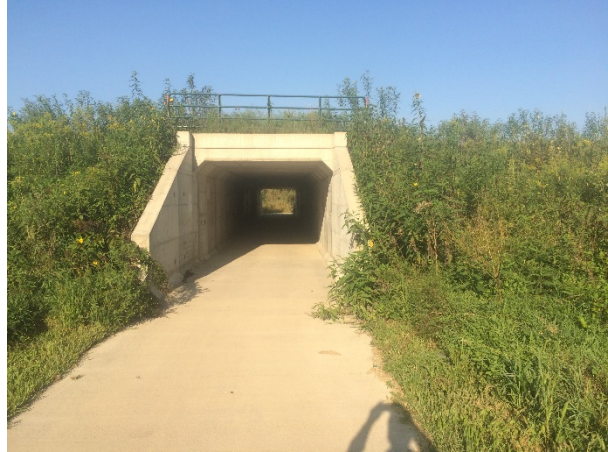
A box culvert underpass for the trail under Highway 63 south of Oskaloosa provides a safe crossing for trail users.
